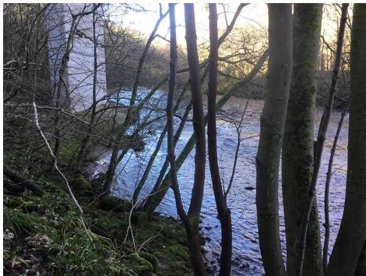
Photograph 1: South pier looking upstream to river training works and position of the new pier
