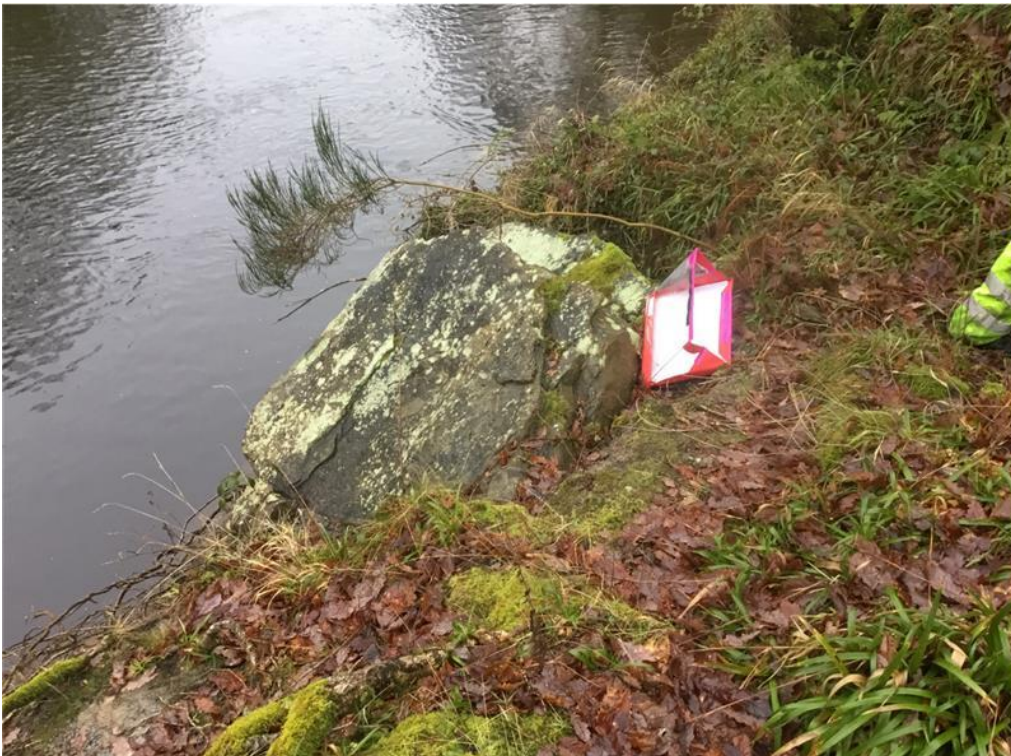
Image 3. Rockfall along northern banks of the River Coquet 200 m downstream of proposed crossing
